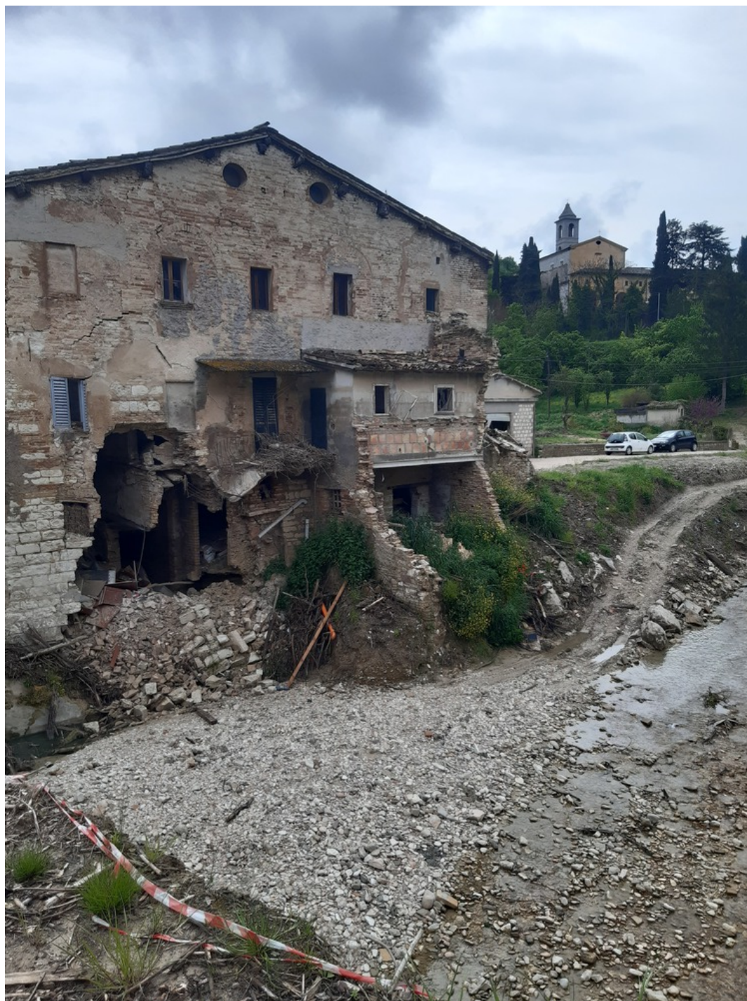
Figure 1: Destroyed house below the city walls of Pergola.*
