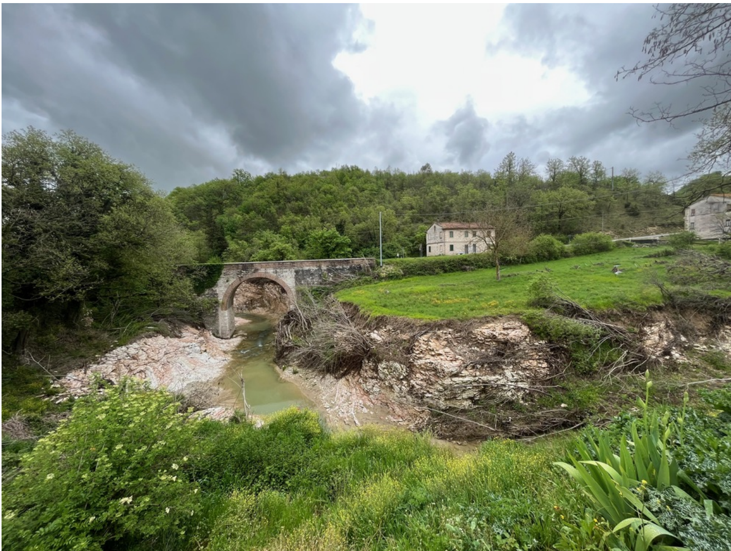
Figure 6: Bridge with one arch which remained intact. On the banks of the riverbed heavy erosion of soil and vegetation, as well as unrooted trees are visible.
