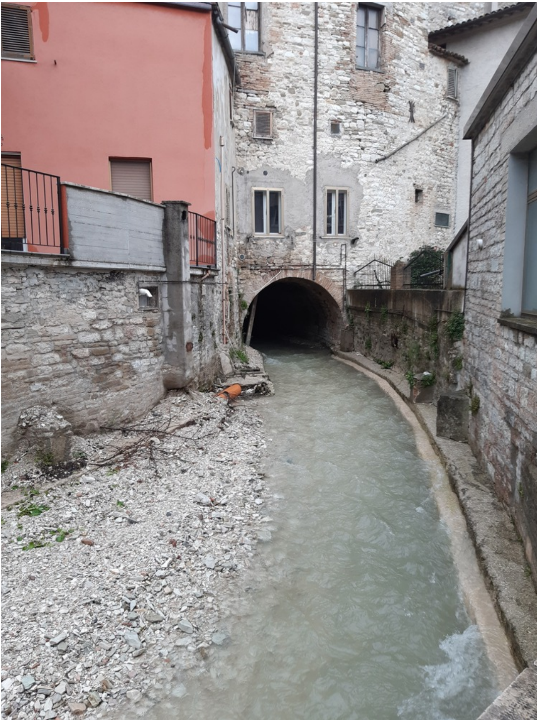
Figure 9: Artifical channel in the city of Cantiano. Spilling over of these channels flooded the whole city center.
