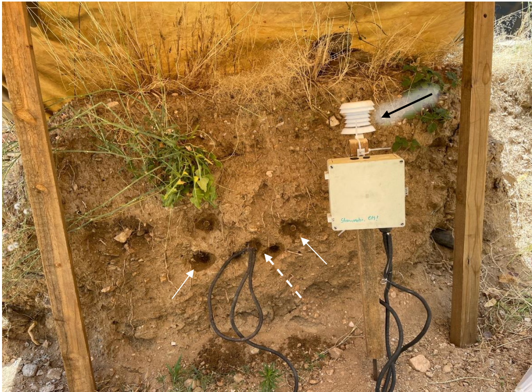
Figure 5. Experiment 2. Installation of the Ec5 with its associated sensors and the two iButtons on a dry soil profile in my garden. The two solid white arrows are pointing to the location of two iButtons which were inserted with the open end of the holder pushed snugly against the soil. The dashed white arrow points to the location of the ECH2O EC5 soil moisture sensor and soil temperature probe. The black arrow points to the solar shade for an air temperature and RH sensor. The latter are fixed above the HOBO Microstation data logger. The dark patches are wet soil, necessitated to allow the placement of the sensors in the hard dry soil. These wet patches dried out within 12 hours. The whole setup was shaded using a small brown polypropylene canvas. This set of measurements were contrasted with a similar setup in soil that was just below field capacity.
